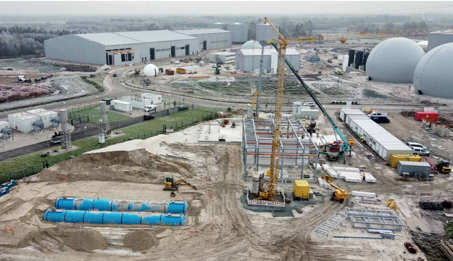
Friesoythe biogas feed-in plant
