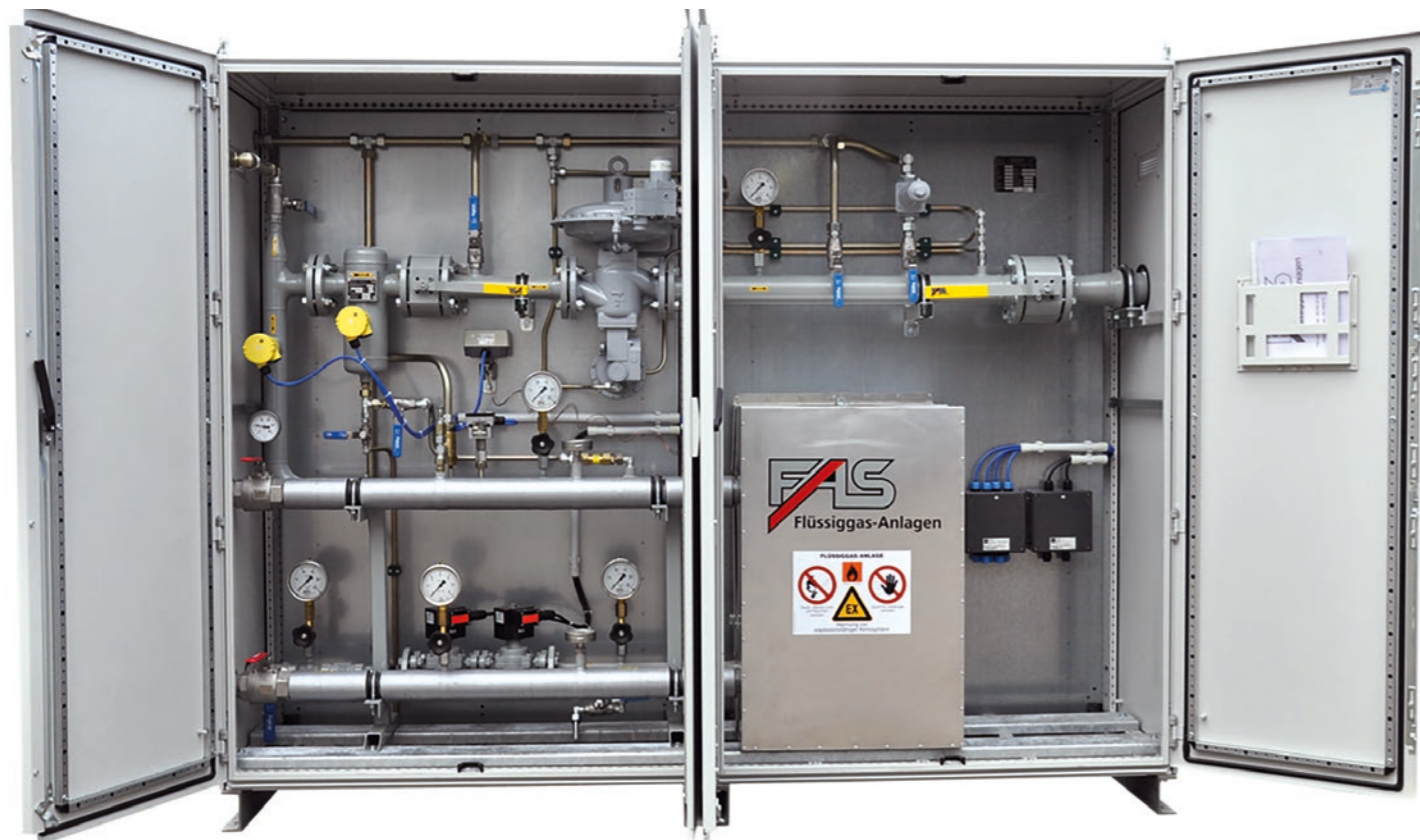
1200kg/h (320 gal/hr) waterbath vaporizer unit in a cabinet with insulated water pipes, liquid trap, electronic level alarms, two stage pressure regulation and over pressure protection with safe gas release.
